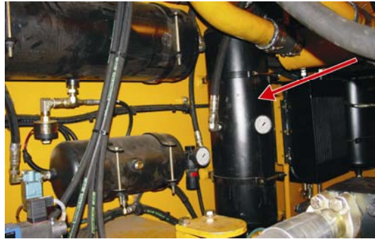
Remove “receiver tank”
